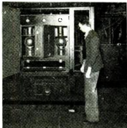
An experimental set-up of the inverter used in the new power distribution system.
